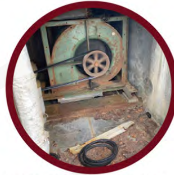
OUTDATED & INEFFICIENT MECHANICAL SYSTEMS
